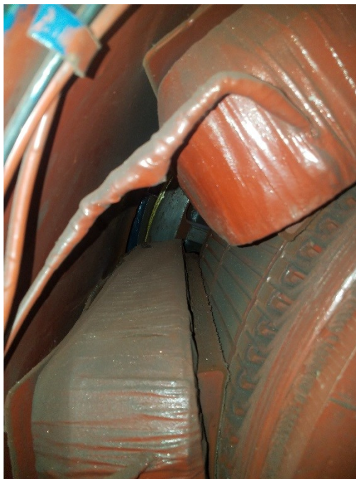
Heavy carbon buildup throughout the machine prior to NitroClean™.
